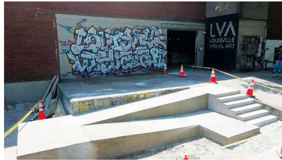
The newly poured exterior steps and ramp at 1538 Lytle Street, LVA's headquarters.
